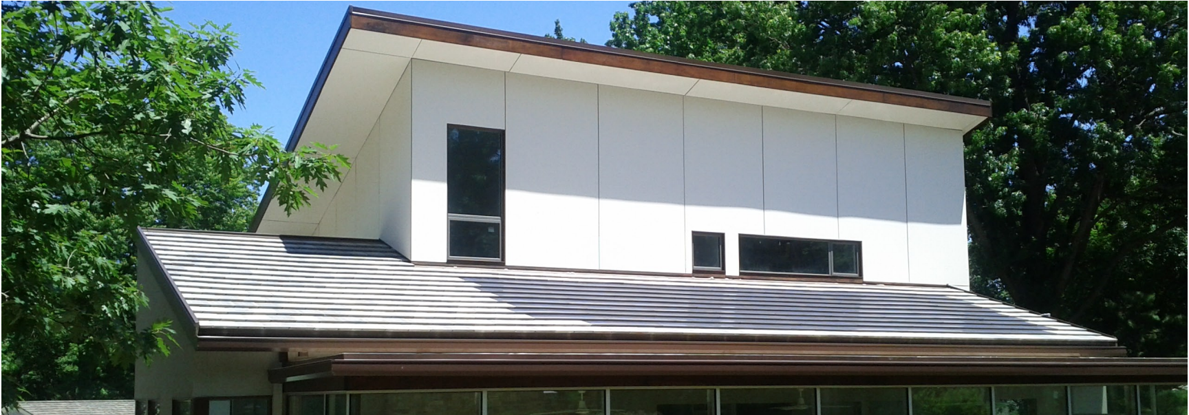
Solar Panels Integrated into a tile roof, Leawood, Kansas
